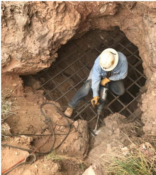
Drilling holes for anchor pins for the rebar grate at the Jarvis Peak Incline.
