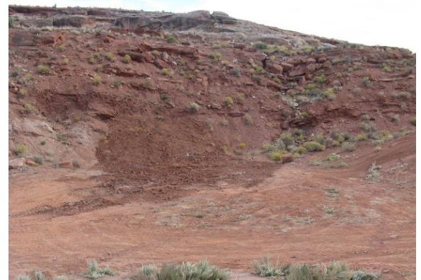
Completed backfill at the Warner Valley Incline. Family memorial to man who died in the mine in 2015.
